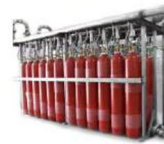
CO2 Extinguishing System
